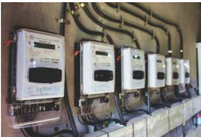
Picture 2: Dhundi cooperative's meter house with individual members' meters and MGCVCL meter
