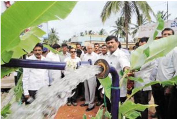
A borewell dug by United Breweries as part of an initiative to provide drinking water to villages in Karnataka.
